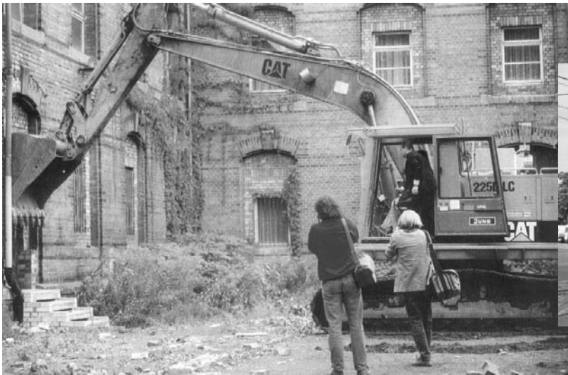
The day the demolition work began, some time in the early/mid 1990's. The last sign of the once big Pinkau factory is gone....
